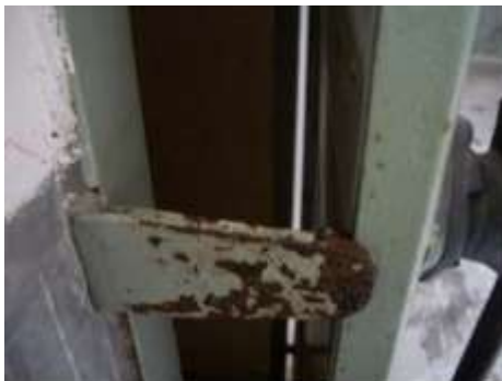
Photo 10: Exit door obstruction.
